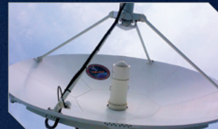
6.1m S & X band ground antenna dish operating 24/7 in full automation, controlled from the SaRC Mission Room.
