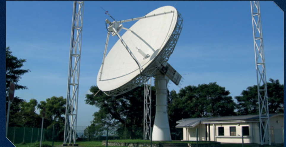
13m diameter tracking antenna with X- and S-band downlink and S-band uplink.
